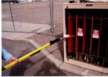
The systemwide phase ID program includes verifying the phase on distribution circuits at APS's underground switching cabinets.
