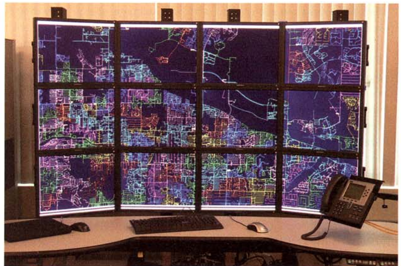
The DOMS will display high-level maps of the entire system or zoom in closer to view a single piece of equipment or a fault on a circuit.
